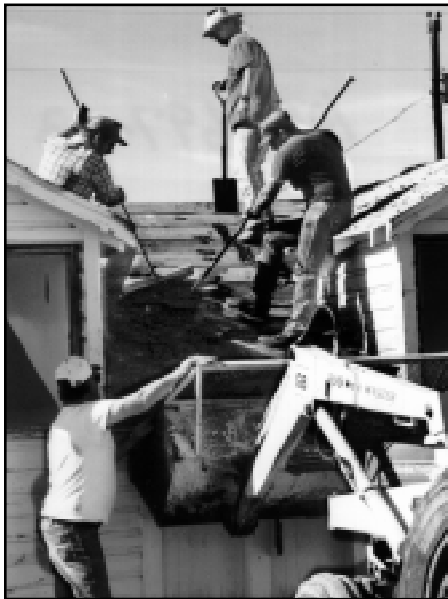
Plant scientist Phil Bruckner (top) and other research center staff pitched in to dismantle a dilapidated building at the research center near Huntley.
